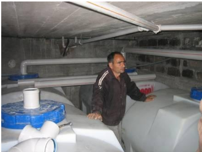
Fig. 11: Urine tanks (4 x 2 m 3 ) in the basement of the school (source: AWHHE, 2006)
