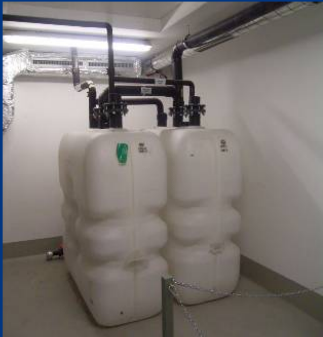
Urine tanks (photo: Otterwasser GmbH)
